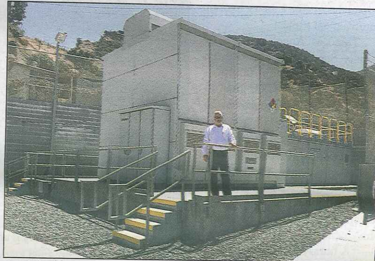
Ron Hite, SCE senior manager of operations in Catalina, stands outside SCE's battery energy storage system.
